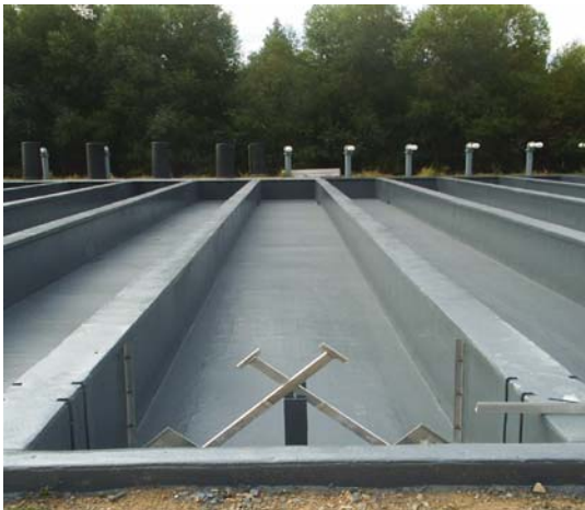
X-Shield FS450 Polyurea was applied 80 mils to concrete channels floor and walls.
