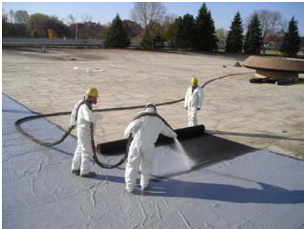
Geotextile fabric rolled over heavily cracked asphalt and sprayed with X-Shield FS450 polyurea coating
