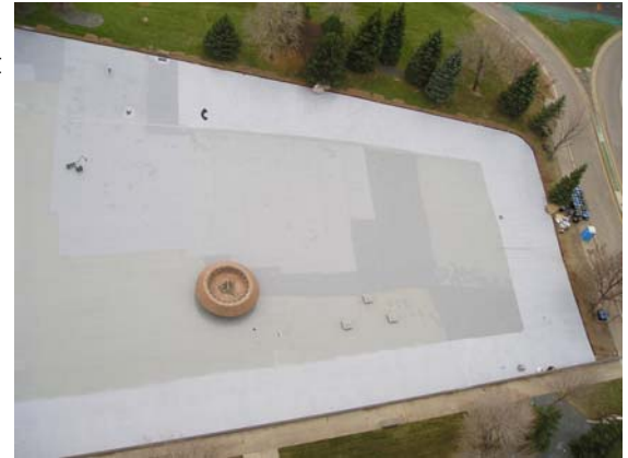
Birds eye view of the new polyurea liner Note: The color stable roller grade polyurea along the edges of the Settling Pond.
