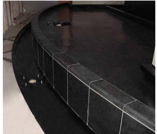
X-Shield FS450 polyurea coating base coat applied to all tough areas and coated with a black aliphatic topcoat X-Shield RG40 to match with existing marble stone.
